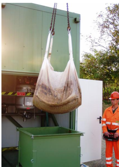
Figure 4 – Dewatered solids removal for dumping after separation from wellstream fluids with a desander.
