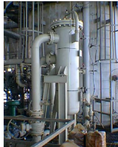
Figure 3 – A 20,000 BPD desander for removing solids >10 \mu\text{m} from the water stream after a production separator.
