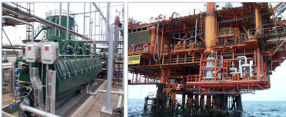
Figure 2. (left) Four-stage mechanical IGF cell installed at a land-based oil facility and (right) a vertical IGF cell (gray vertical vessel near center) installed on an offshore fixed-platform.
