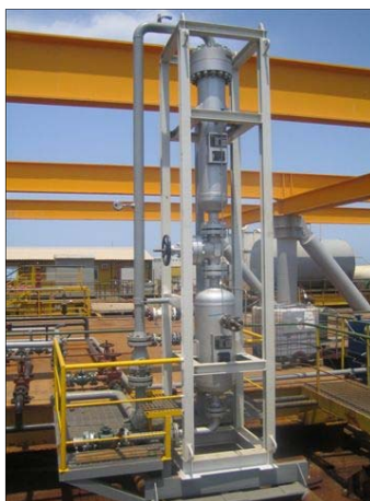
Figure 4 – Photograph of 900# wellhead desander system installed on shallow platform in Caspian Sea.
