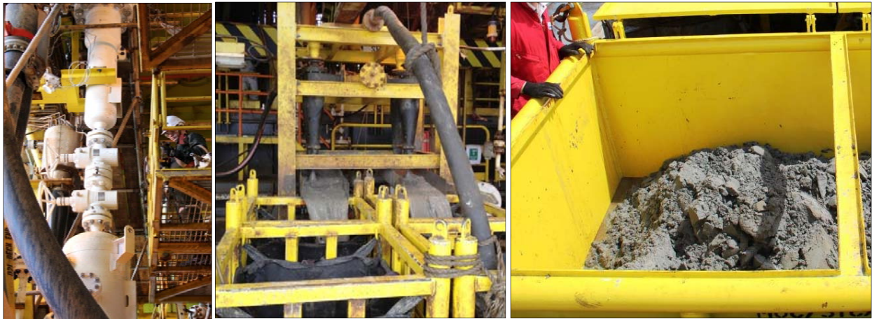
Figure 6 – (left) 1500# wellhead desander integrated into the deepwater spar well bay, (middle) solids collection and dewatering station, and (right) collected solids transported by skip to landfill disposal.
