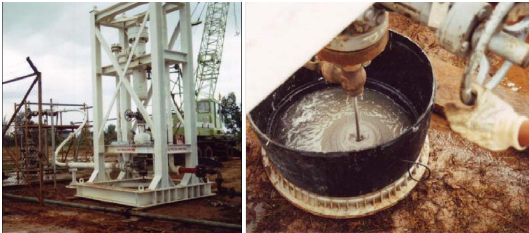
Figure 5 – Photographs of a 900# portable wellhead desander installed on gas wells onshore Indonesia.
