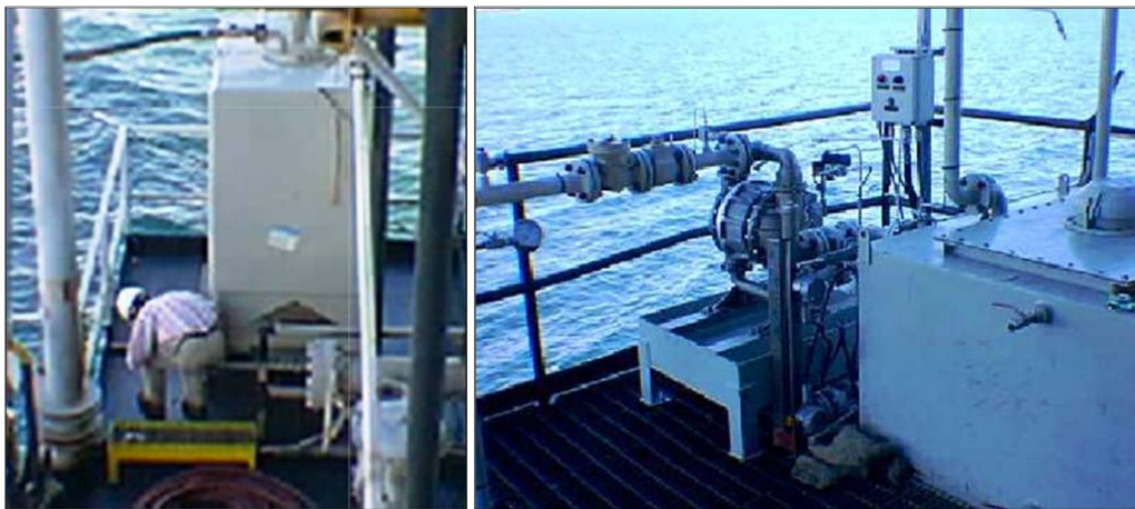
Figure 9 Dewatering and transport station receiving slurry from produced oil and water desanders on fixed leg facility. Photos show (left) dewatering bin for vapor containment and (right) liquid collection and pumping station.
