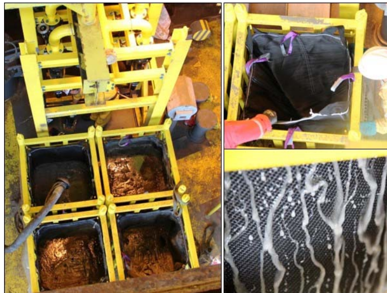
Fig. 3 – Two-stage open dewatering system employed on deepwater spars in the South China Sea. Bulk dewatering employs a bank of urethane cyclones (left picture, upper portion) and four-place hanging dewatering bags (left picture, lower portion). The support of the dewatering bag is shown in the upper right photo, while the liquid filtrate removal process is shown in the bottom right photo.
