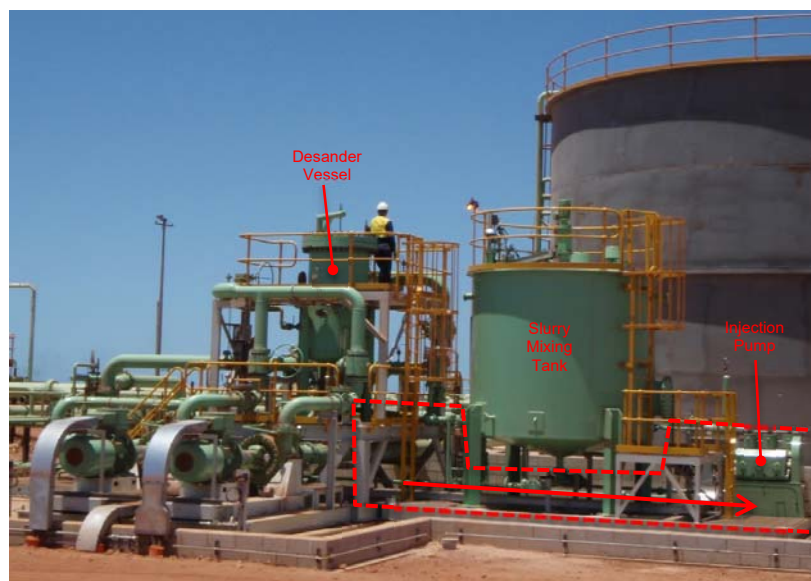
Fig. 7 – Transport of slurry from a produced water desander to an injection pump in an onshore Australian application.
