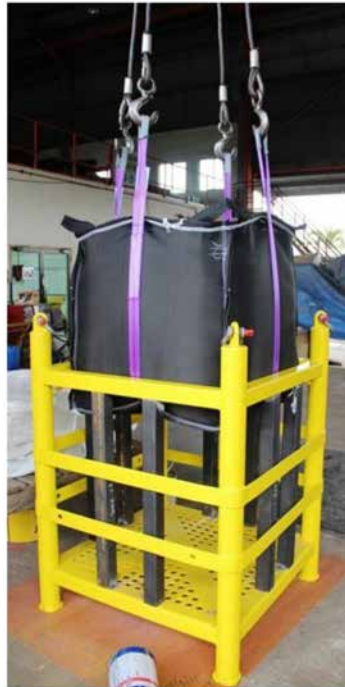
Figure 5—Dewatering filter bag (left photo) being lifted from a simple support frame.
