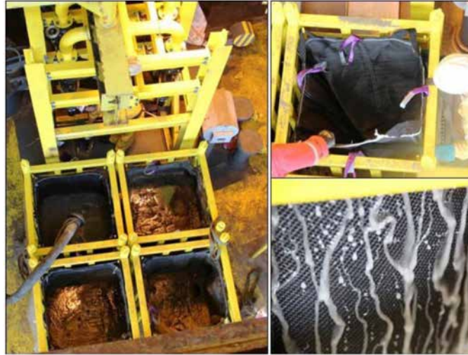
Figure 3—Two-stage open dewatering system employed on deepwater spars in the South China Sea. Bulk dewatering employs a bank of urethane cyclones (left picture, upper portion) and four-place hanging dewatering bags (left picture, lower portion). The support of the dewatering bag is shown in the upper right photo, while the liquid filtrate removal process is shown in the bottom right photo.
