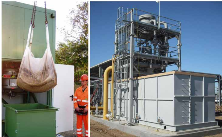
Figure 8—(left) Crane lift of a dewatering bag after filling with solids from a multiphase desander and (right) truck roll-off container to collect solids directly discharged from a produced water desander.
